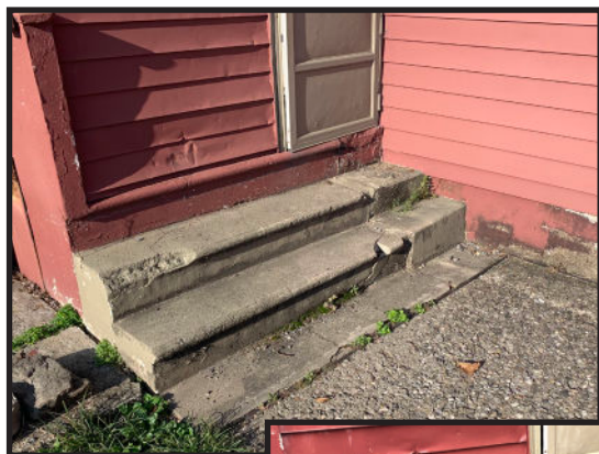
Before - Cracked Concrete Steps
